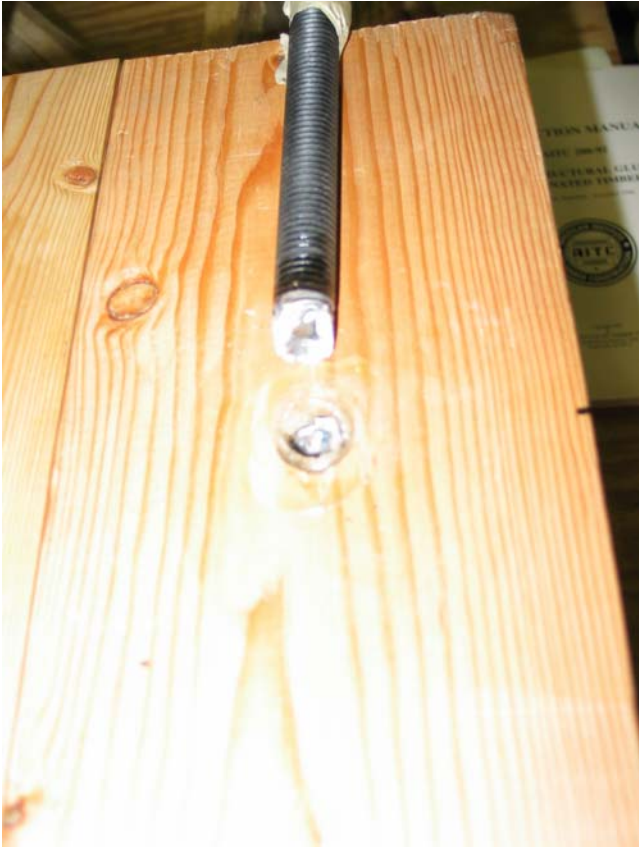
Figure 3: Weld failure between rebar and threaded rod.
